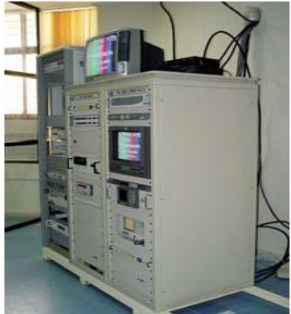
SATCOM Earth Station Controller
